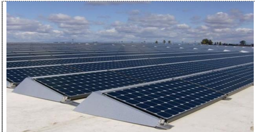
Figure 1. General view of a solar photovoltaic station with a capacity of 20 kW
