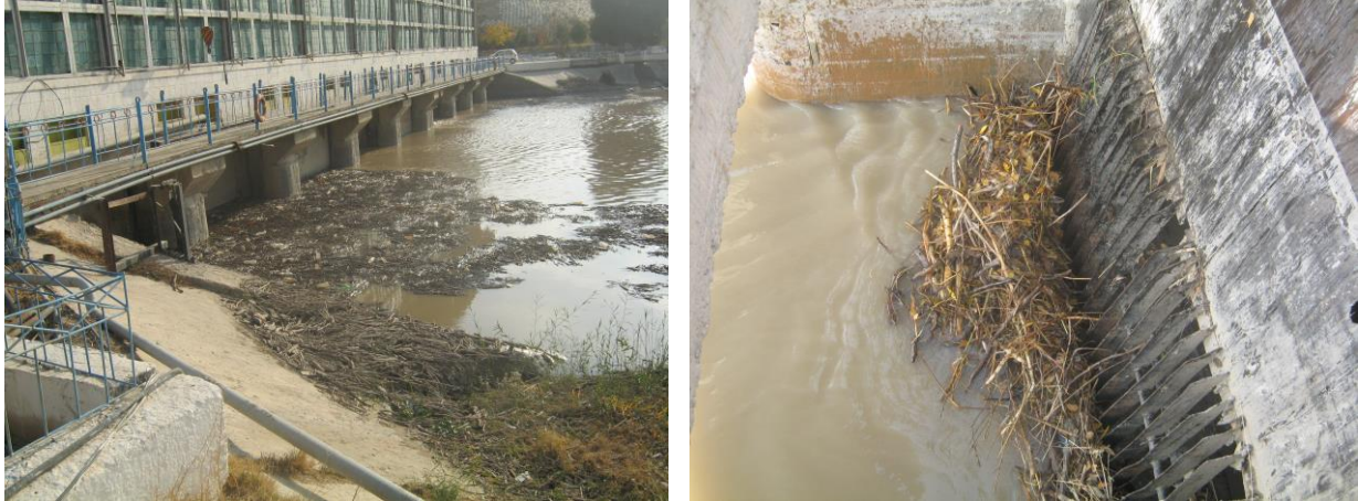
FIGURE 1. Accumulation of driftwood and silting of slopes in the front chamber of the PS "Amu-Bukhara 1" Amu-Bukhara machine channel.
