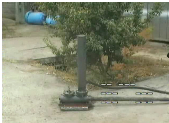
Figure 1. Sample of the pumping installation
