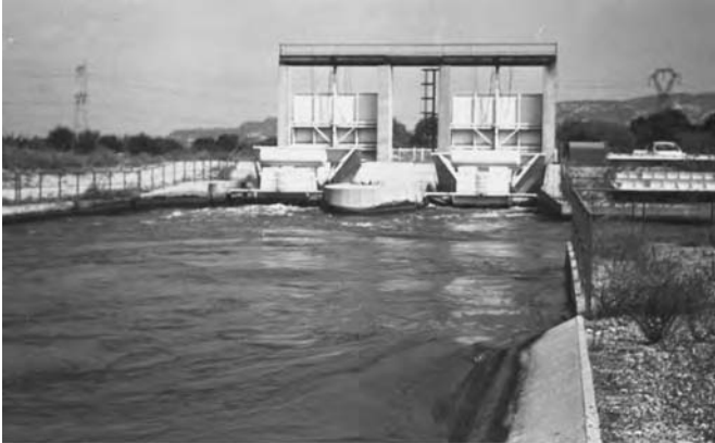
(a) Discharge regulator in a canal system in France
