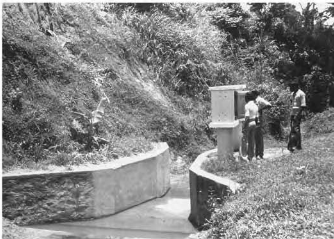
(b) Parshall flume
