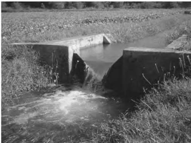
(c) Photograph of a V-shaped weir
