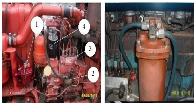
Figure 8. Installation of diesel fuel and bioethanol liquid heating transfer device in the system. 1-rough cleaning filter; 2-low pressure fuel suction pump; 3-high pressure fuel pump; 4-temperature stimulator.
