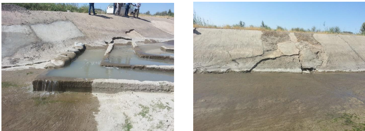
Picture 1.4. Disorders in the lower Amu-Zang canal in Surkhandarya region.
