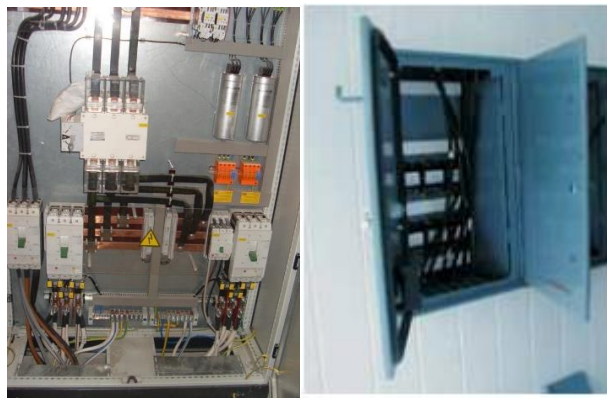
3.11-rasm. Kontroller shkafi kiritish va chiqarish modullari bilan
