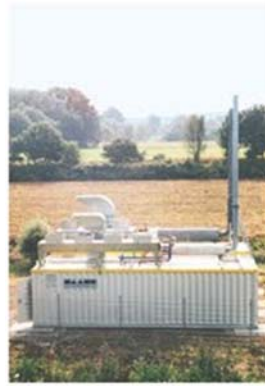
Container-CHP in Borken
