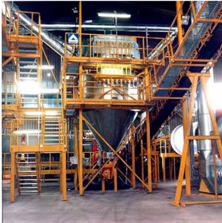
Hot gas filter of the pyrolysis plant of the BRZ company in Herne
