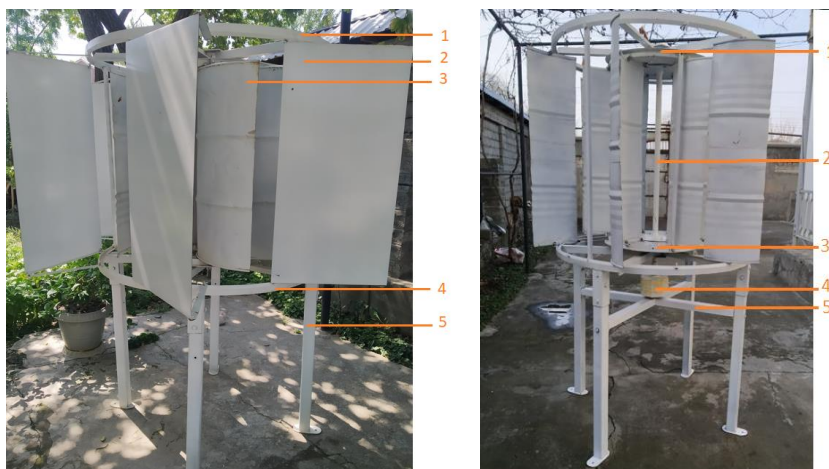
Fig. 4. Wind power plant. 1,4 - rings that hold the guide wings; 2 - guide bars; 3 - working wheel blades; 5 - holding legs; 6,7 - discs holding the main wings; 8 - generator; 9 - frame holding the generator; 10 - shaft
