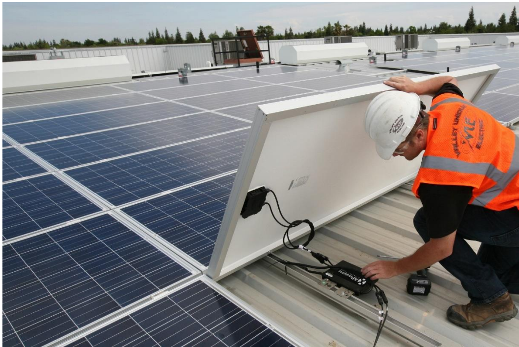
Figure 4.9. Microinverter mounted on the back of the solar panel
