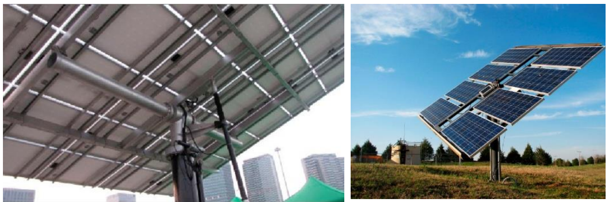
Figure 3.21. Two-axis tracker solar power station
