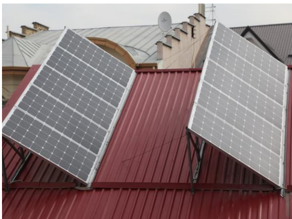
Figure 3.12. The position of the solar module device installed on the roof of the House
