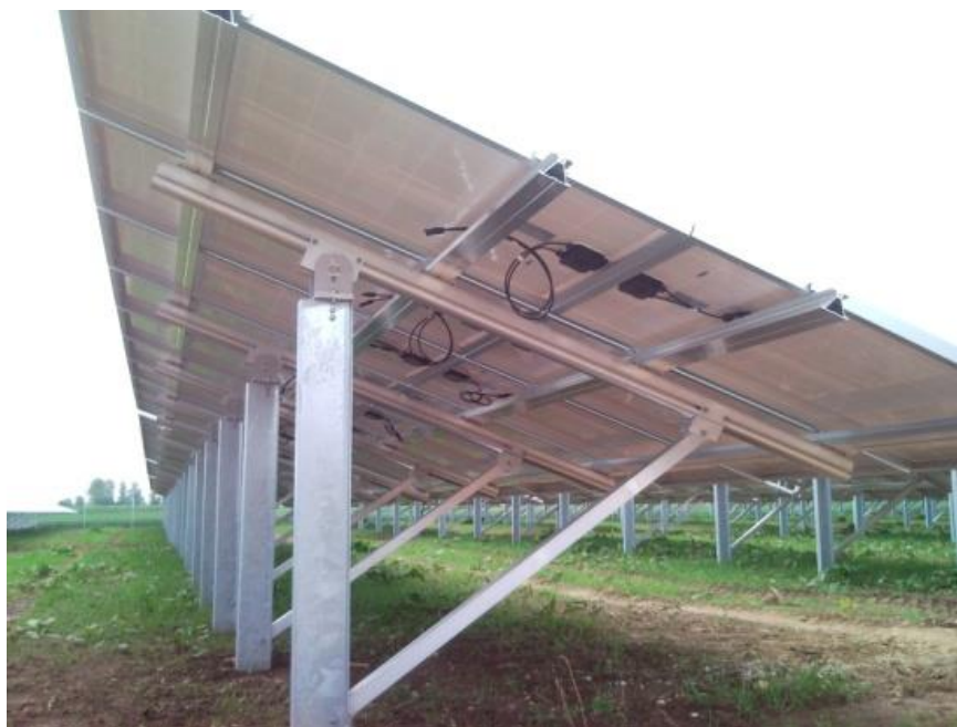
Figure 3.20. One-axis tracker solar power station
