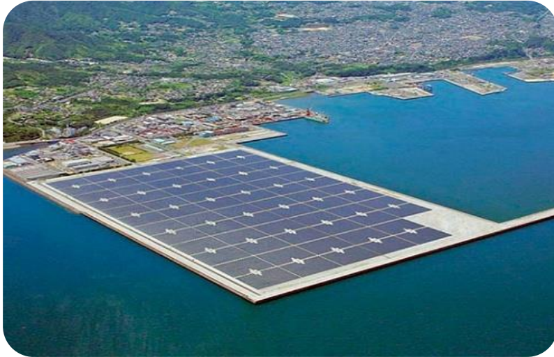
Solar panels installed in Japan
