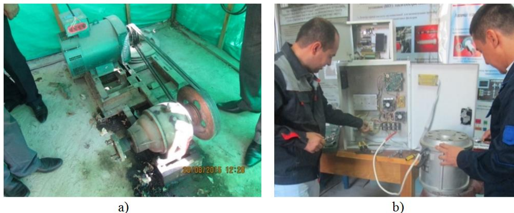
Figure 4. Place of installation of the generator and reducer of the device (a) and the process of preparation of the generator and power unit for operation (b)
