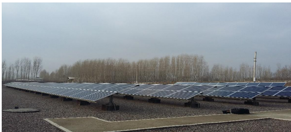
Figure 1. Pop solar power plant
