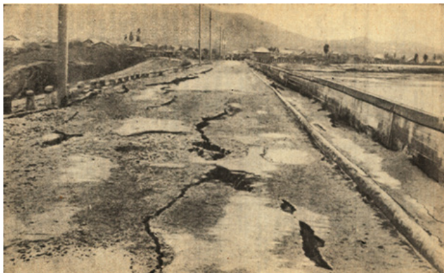
Fig. 2. Damage to the dam of the Chiryurt hydroelectric power station during the Dagestan earthquake on May 14, 1976
