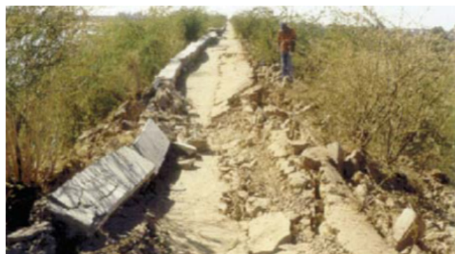
Fig. 1. Longitudinal fractures on the upstream slope of the Feitigadh dam (India) caused by the Bhuj earthquake on January 26, 2001
