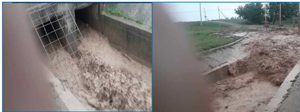
Fig. 3. Faults in the drainage structure after the flooding of the Langar flood reservoir
