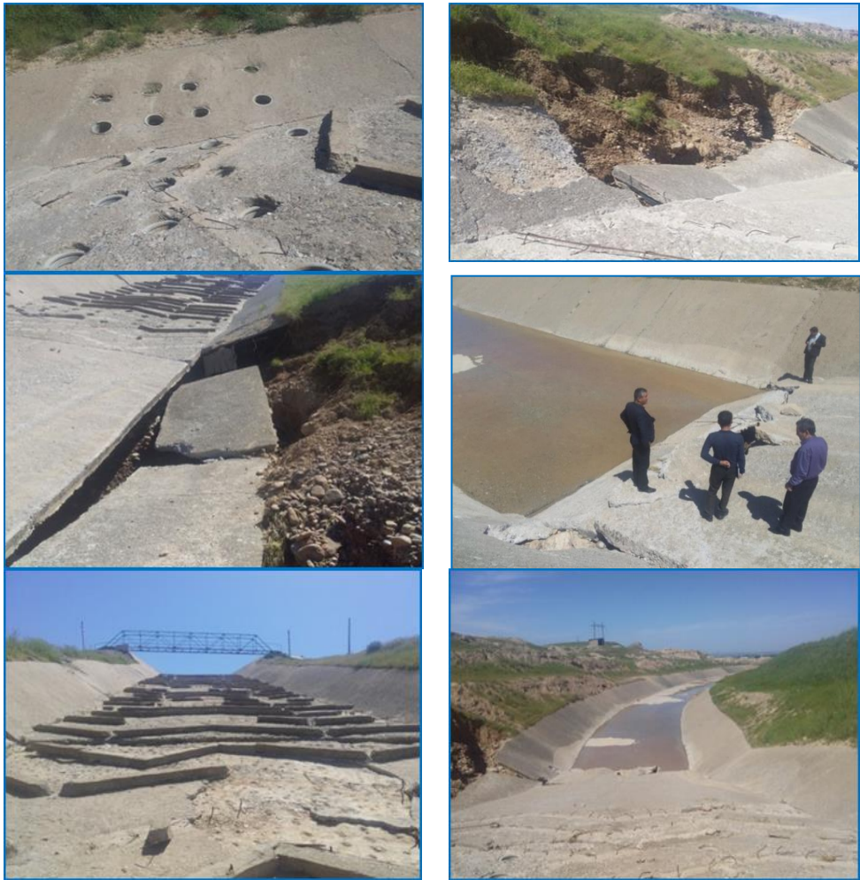
Fig 2. Damage caused by floods at the Langar flood reservoir
