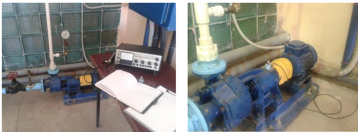
Fig. 5. Option to install vibration sensor on cantilever centrifugal pump NL125 / 200-72
