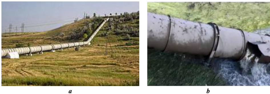
Fig. 1. Culverts [4, 16]: a is in the Crimea near the city of Simferopol; b is in Ingushetia on the Alkhanchurt canal with a pipe defect, 2019
