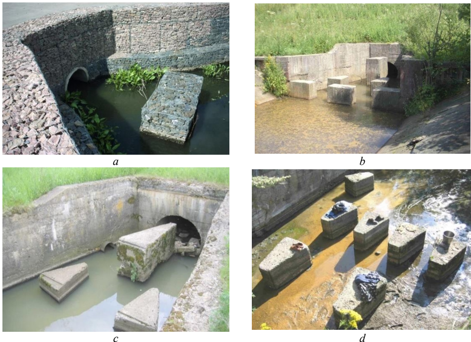
Fig. 1. Results of tubular culverts surveys held in Moscow Region, built according to standard designs of different years [3,5] (photo by the authors): a is deformation of fastening of downstream of single-point tubular crossing from corrugated pipe and gabion structures on Moscow-Kolomna highway, 2021; b is water well with dampers-spreaders behind two-point spillway of pond on river Chernichka in Podolsk region in 2009; c is fragments of building structures in pipe and at beginning of water well of dam on river Solovka, Podolsky district, 2019; d is displacement of absorber of second row of Ptitsegradsky pond on river Torgoshe, Sergiev Posad district, 2005.
