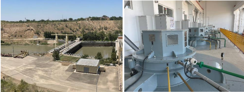
Figure 1. Reconstruction of the fore chamber of the hydroelectric complex of the PS "Kiziltepa" and the engine room of the PS "Kuyumazor" with new Chinese equipment
