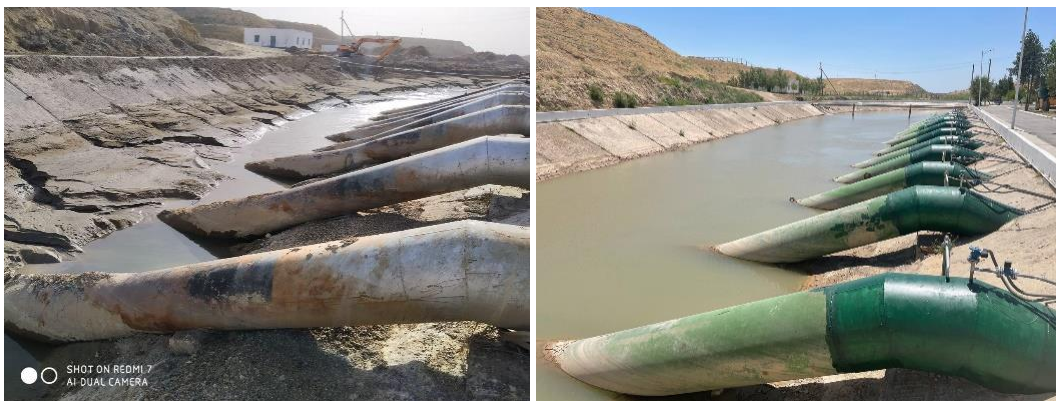
Figure 2. Reconstruction of suction pipelines (2022 compared to 2020) and cleaning of the water intake of the PS "Kiziltepa-1"
