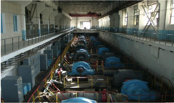
Fig. 1. Engine room of the Kiziltepa 2 pumping station.
